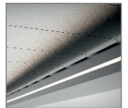
LED lighting - LED strip lights, integrated with the gutter
