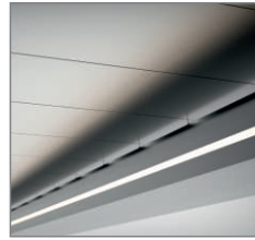
LED lighting - LED strip lights, integrated with the gutter
