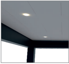
LED lighting - spotlights
